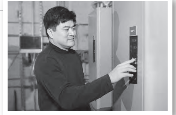
"These boilers have an operating design efficiency of up to 98%. Together with an electronic EMS and energy-efficient pumps, we anticipate significant energy savings."
