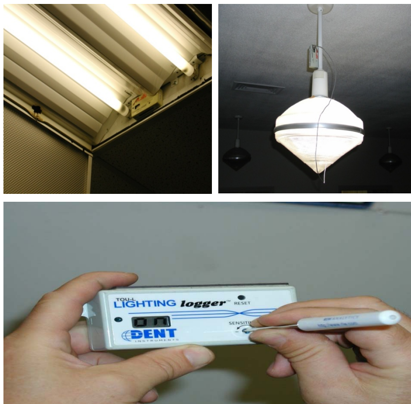
Figure 8-2: Lighting Logger Installation and Calibration
