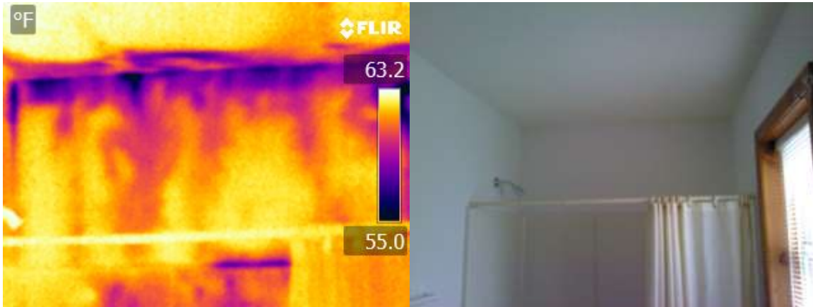
Figure E-18: Likely Moisture Damage in Bathroom
