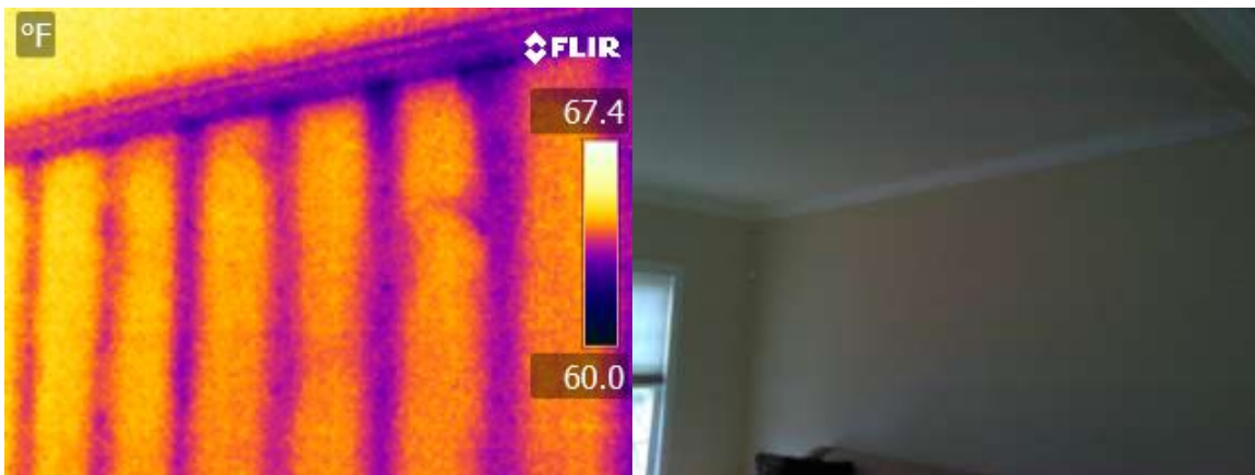
Figure E-22: Well Installed Wall Insulation
