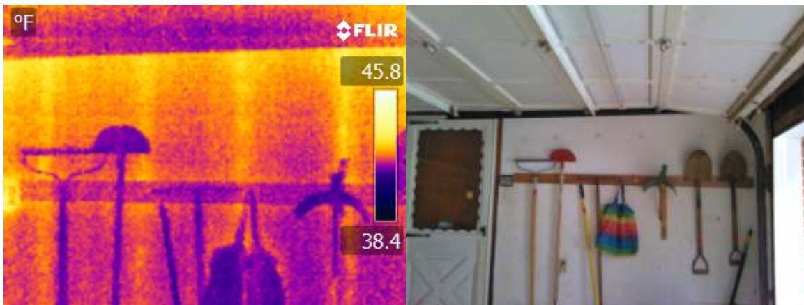
Figure E-15: Settling of Blown-In Cellulose Insulation
